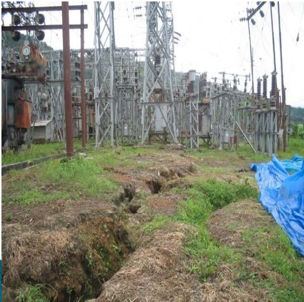
Land Sinking at Zuangtui Power Sub-Station
