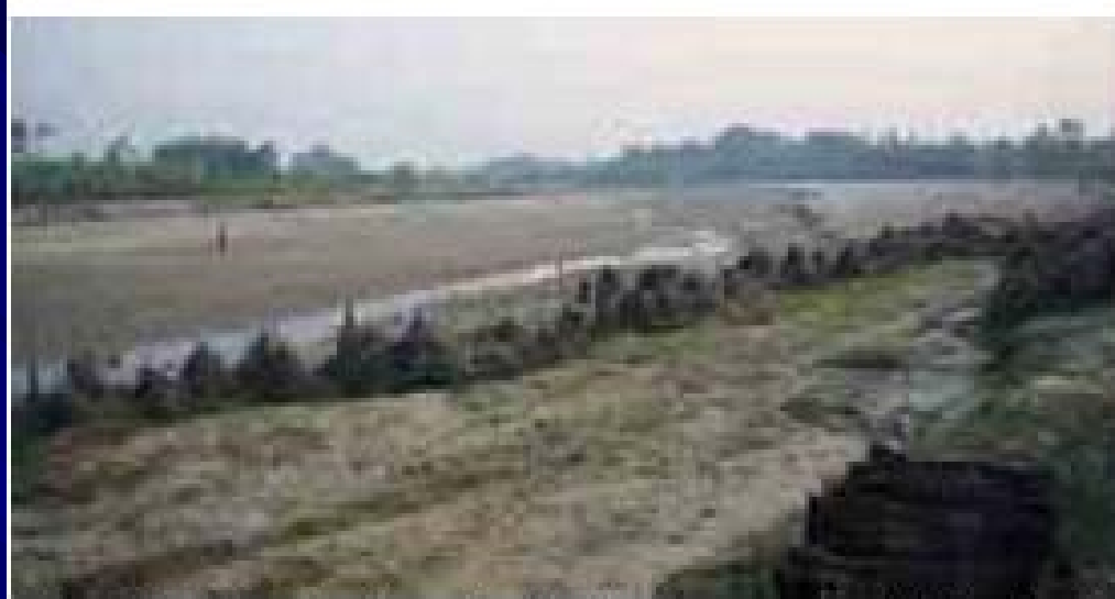
Figure 19: Embankment made out of bamboo constructed by a local NGO using local knowledge and local material. Phoolparasi VDC, Sarlahi District
