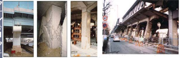
Damages of Railway Facilities of Kobe City
