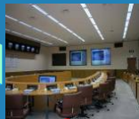
Emergency Relief Headquarters Control Room
