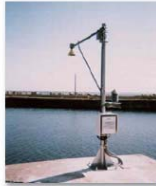
◆ Acoustic Type Gauge Station
