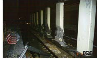
Damaged columns in the subway station, 1995 Kobe earthquake
