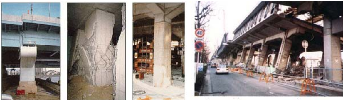
Damages of Railway Facilities of Kobe City
