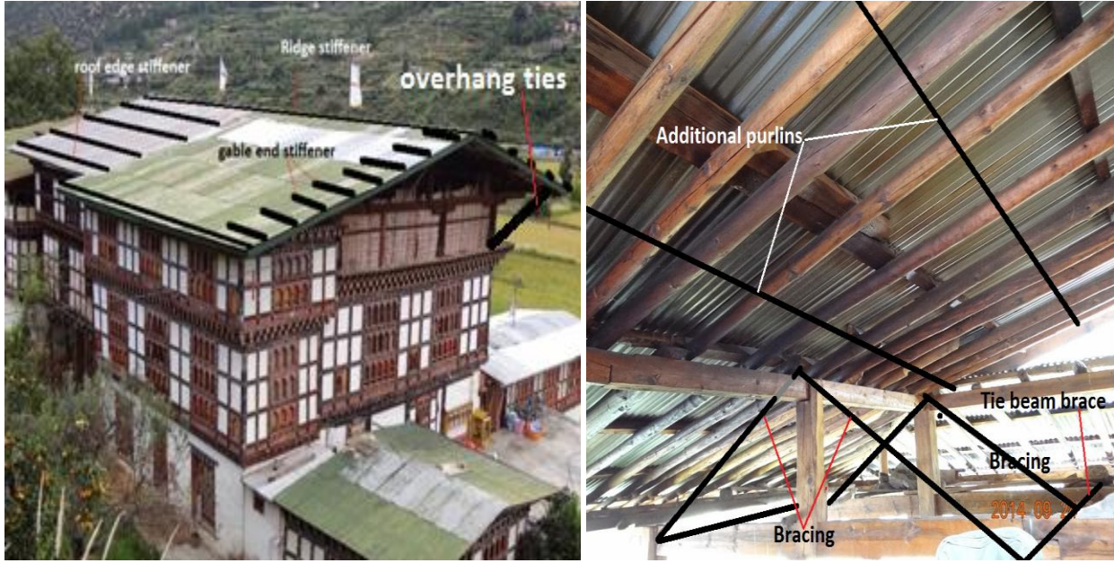
Figure 62: Gable end stiffener, roof ridge stiffener, corner stiffener and overhang ties (L) and additional purlins & bracing (R)
