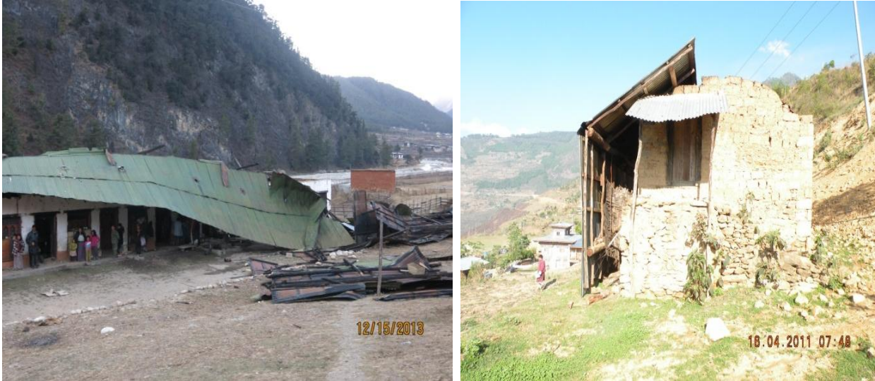
Figure 51: Sliding of roof (L) and over-turning of roof (R)
