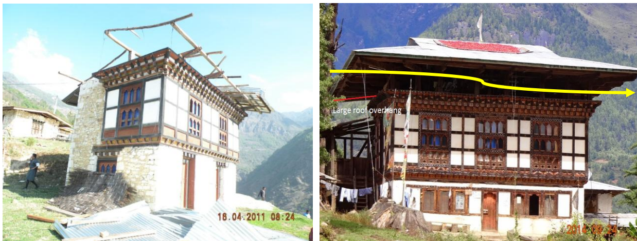
Figure 49: Gable roof end failure (L) and large roof overhang (R)
