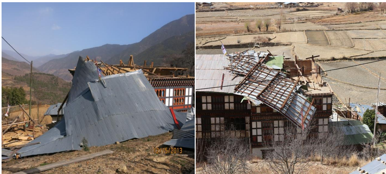
Figure 45: Failure due the poor connection between rafters and struts causing full-blown off
