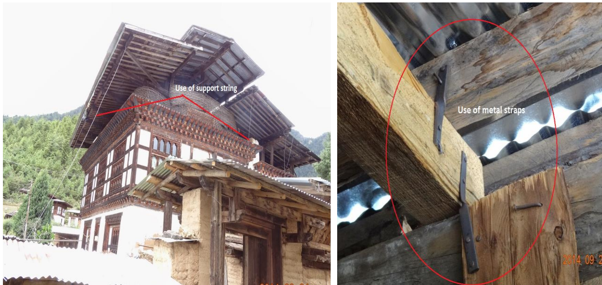
Figure 59: Use of support string (L) and metal straps (R) during the reconstruction in Paro
