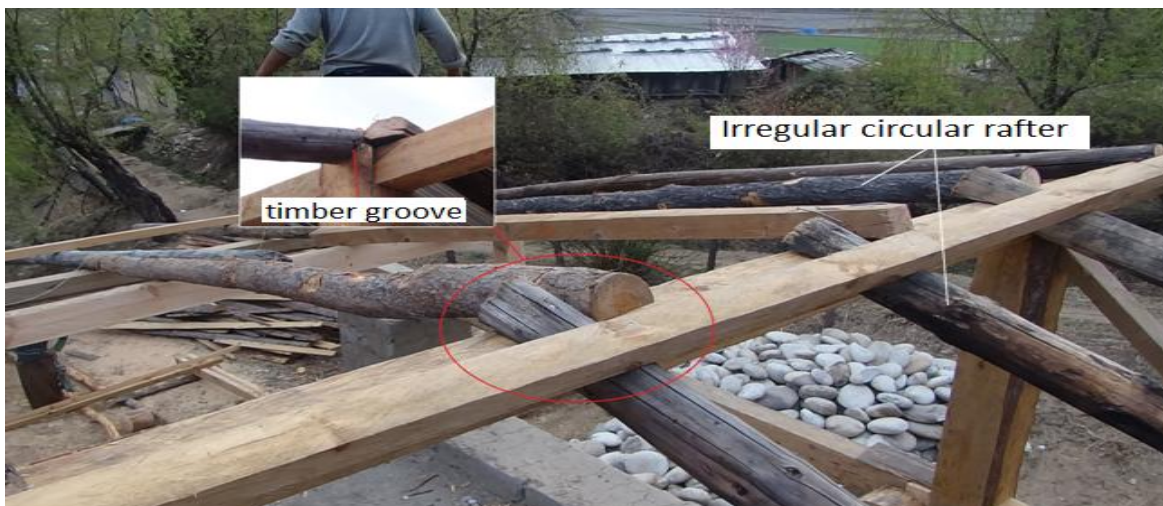
Figure 44: Roof ridge connection in rural home roof with deep groove and lap joint
