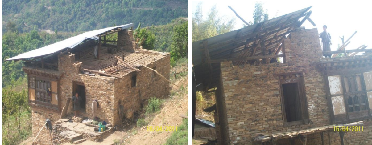
Figure 43: Roof ridge failure during 2011 windstorm
