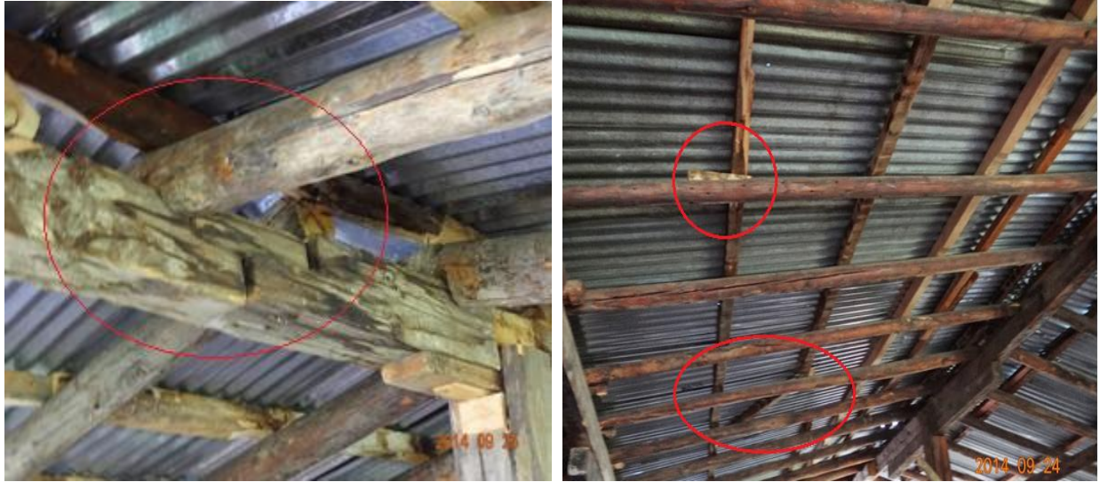
Figure 48: Weak lap joint at roof ridge (L) and purlin are not laid equally (R)
