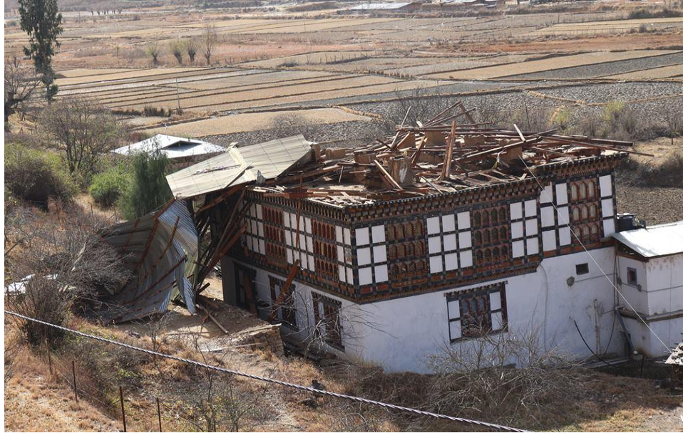
Figure 46: Full-blown of rural home roof due to failure in the connections
