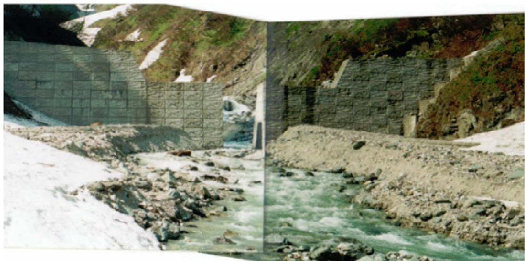
Fig. 119. Sediment originally trapped upstream of the slit dam, released during the recession period, and deposited again downstream of the sabo dam.
