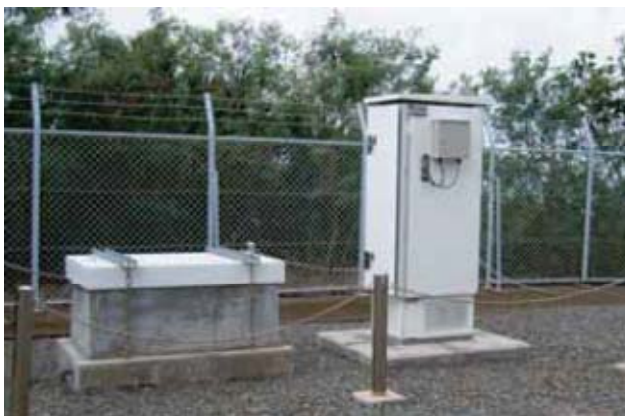
Fig. 28. Communication Facilities in Shelter
