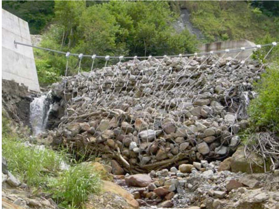
Fig. 120. Debris flow barrier successfully catching the debris flow snout at Mount Tateyama, Japan. Part of the wire (left) was cut by boulders.
