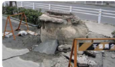
2011: Great East Japan Earthquake; damage to a manhole in the Takasu District, Urayasu City (Institute of Scientific Approaches for Fire & Disaster)
