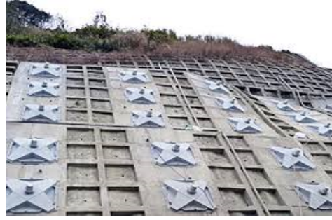
Reinforcement solutions against landslide by metal rock anchor combined with collecting groundwater
