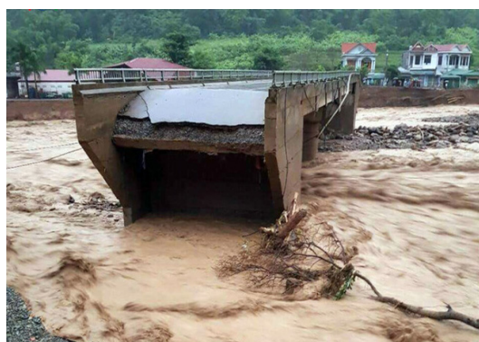
Nam Pam (Son La) Bridge was broken in the flash flood on August 3 - 8, 2017
