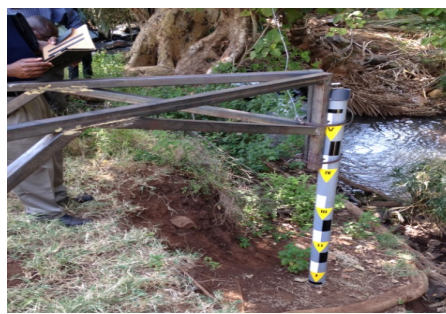
Installation on a metal fabricated stand (Kenya)
