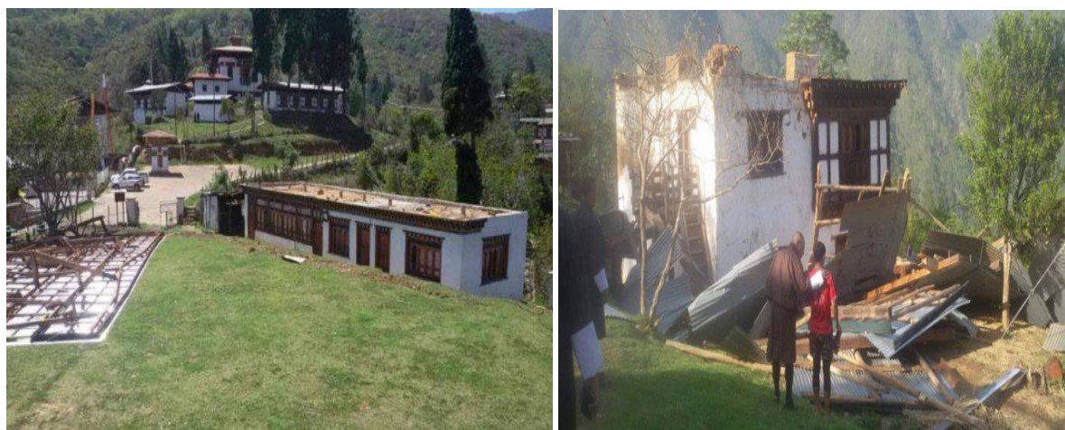
Figure 10: BHU and Rural home roof damage by windstorm
