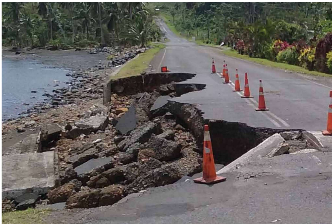
Figure 8: Damage to roadway in Cakaudrove Province on Vanua Levu post Cyclone Winston 2016
