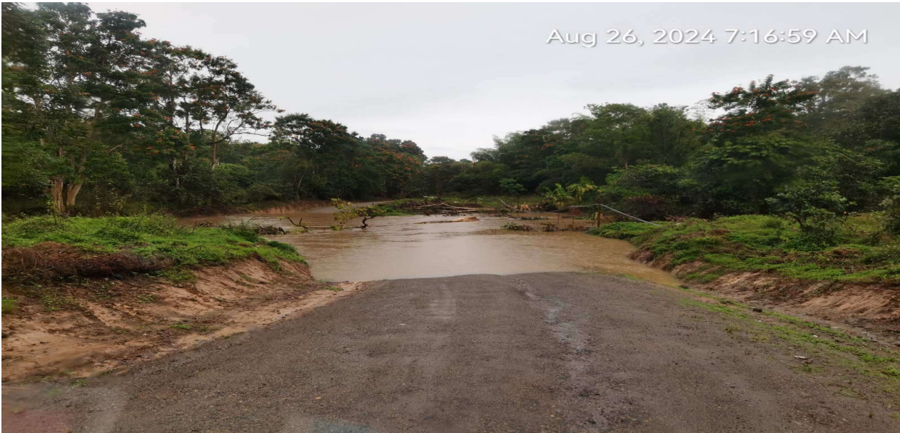
Figure 6: Flooded access road during the August Floods 2024 (source: NDRMO Fiji)
