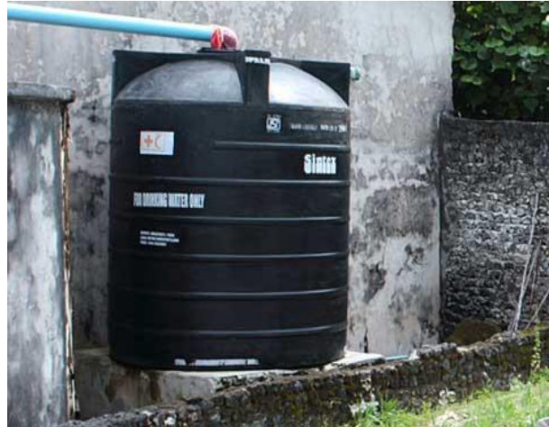
FIGURE 22: PUBLIC WATER TANK
