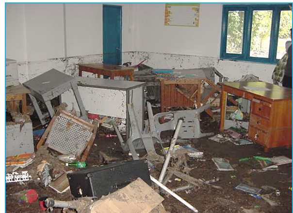
FIGURE 16: AFTERMATH OF 2004 TSUNAMI (CLASSROOM DAMAGED)
