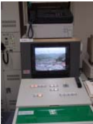
Tsunami Observation System, Taro
