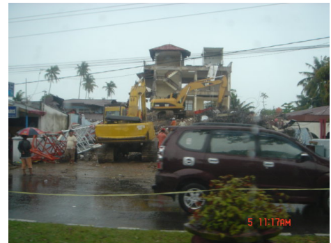
[Collapsed multi-story building]
