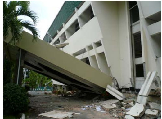
[The first floor collapsed in the Padang Earthquake of October 2009.]
