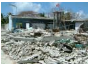
Collapsed Building in Vilufushi Island, Thaa Atoll
