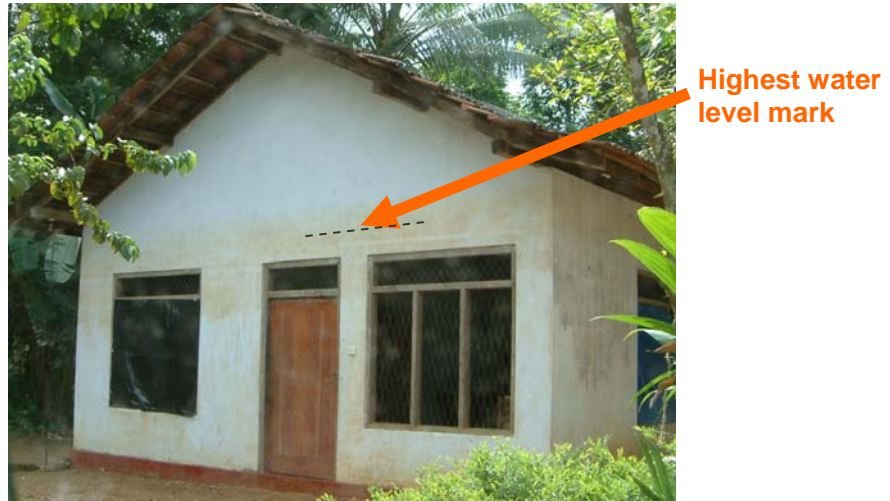
Fig. 4-2-2-3 A house with the highest water level marked on its wall
