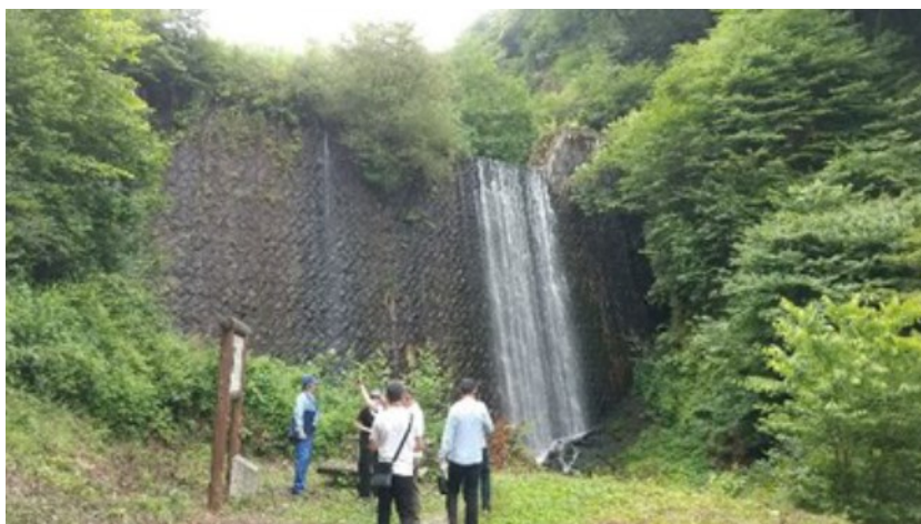
Figure 4.6 Site visit to Sabo facilities along the Karasu River Basin in Gunma Prefecture
